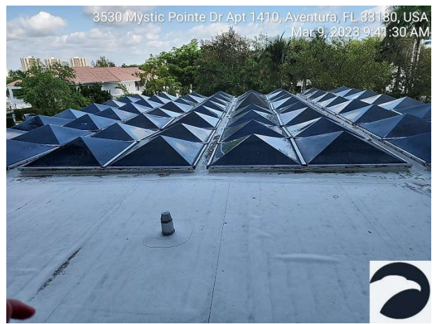
Photo 6. Existing roofing system at Porte cochere to be replaced
