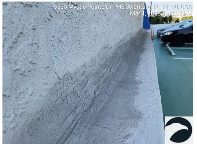
Photo 12. Horizontal expansion joint to be replaced.
