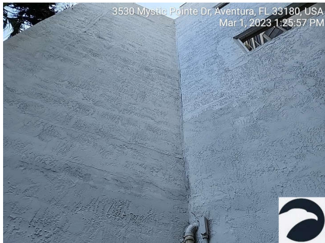
Photo 11. Vertical expansion joint to be replaced.
