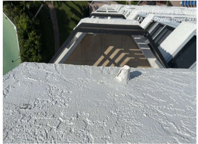
Photo 8. Scuppers to be replaced.
