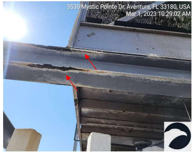
Photo 7.7.12 – Mild corrosion at the cooling tower supports (Main Roof)
