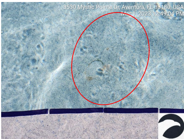
Photo 7.8.13 – Deteriorated finish surface at jacuzzi (Pool Deck Level)
