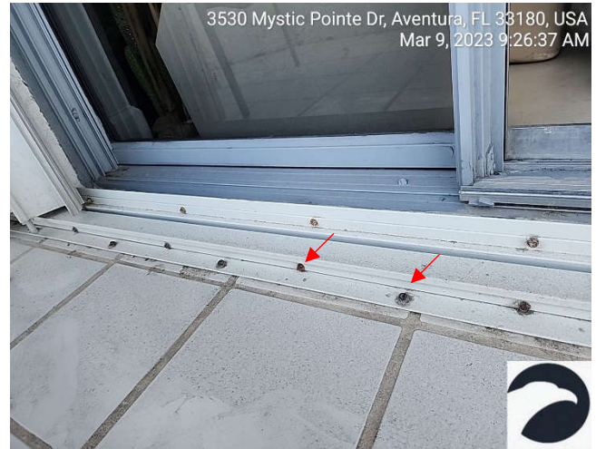
Photo 7.3.c.2 – Corroded anchors of the accordion shutter at sill track (Unit 1418)
