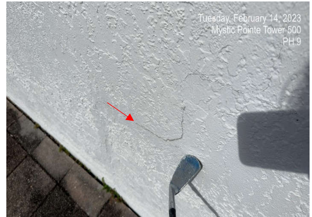
Tuesday, February 14, 2023 Mystic Pointe Tower 500 PH 9 Photo 7.2.c.24 – Cracked stucco and hollow sound at parapet wall (Unit PH 09)
