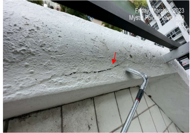
Photo 7.2.c.16 – Cracked stucco with hollow sound at balcony knee wall (Unit 903)
