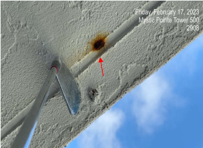
Photo 7.1.b.5 – Rust spot at the balcony ceiling (Unit 2908)
