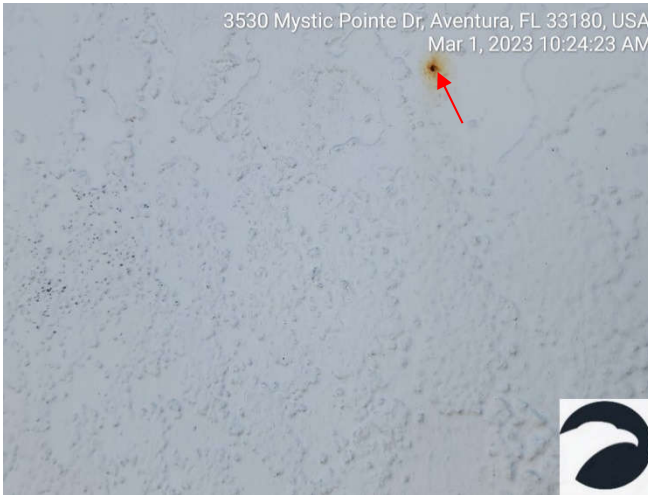
Photo 7.1.b.19 – Rust spot at parapet wall (Roof Level)
