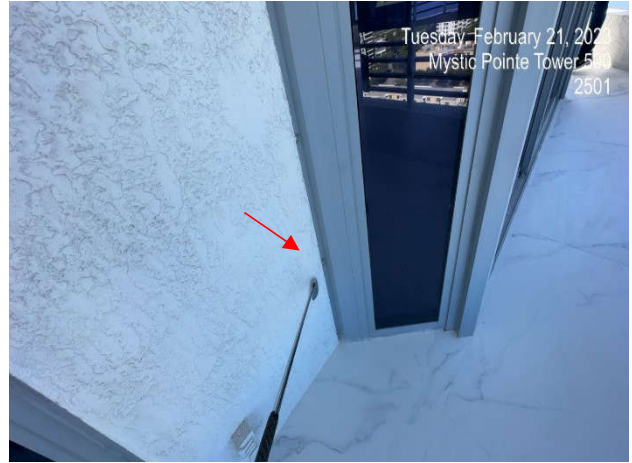
Photo 7.2.c.4 – Hollow sound and stucco delamination at balcony wall (Unit 2501)
