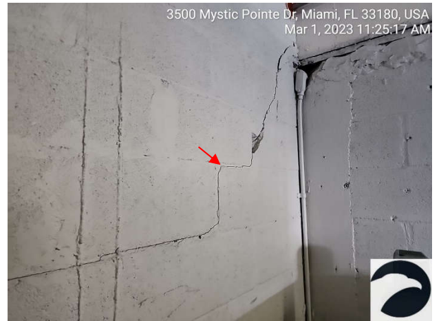
Photo 7.1.c.4 – Stair-step crack at exterior CMU parapet wall of the Emergency Generator Room (Ground Level)
