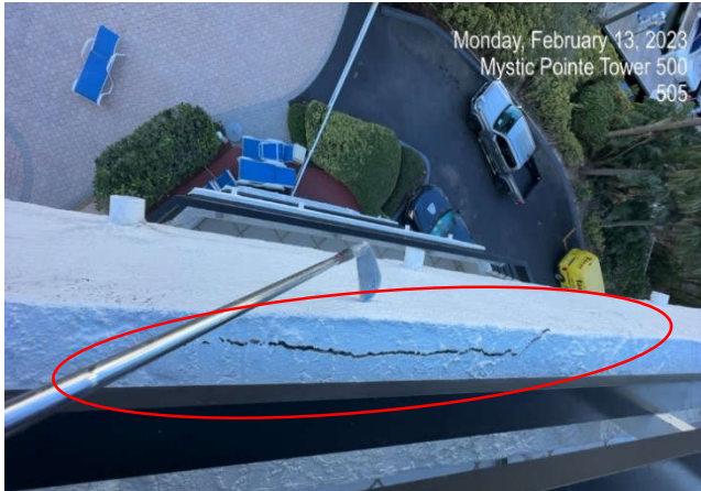
Photo 7.1.a.11 – Cracked concrete and hollow sound at balcony knee wall (Unit 505)
