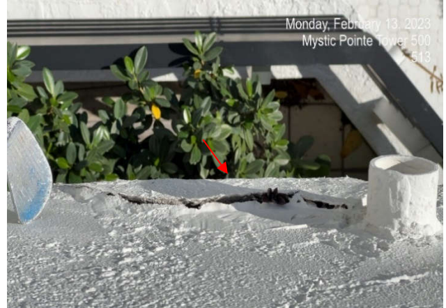
Monday, February 13, 2023 Mystic Pointe Tower 500 513 Photo 7.1.c.22 – Cracked stucco and evidence of biological growth at balcony knee wall adjacent to the scupper (Unit 513)
