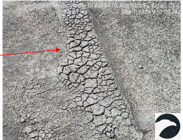
Photo 7.7.6 – Deteriorated and cracked roofing membrane (Main Roof)
