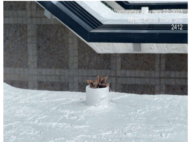
Photo 7.5.2 – Biological growth at scupper (Unit 2412)
