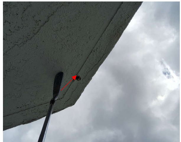
Photo 7.1.b.2 – Rust spot at the balcony ceiling (Unit 2010)
