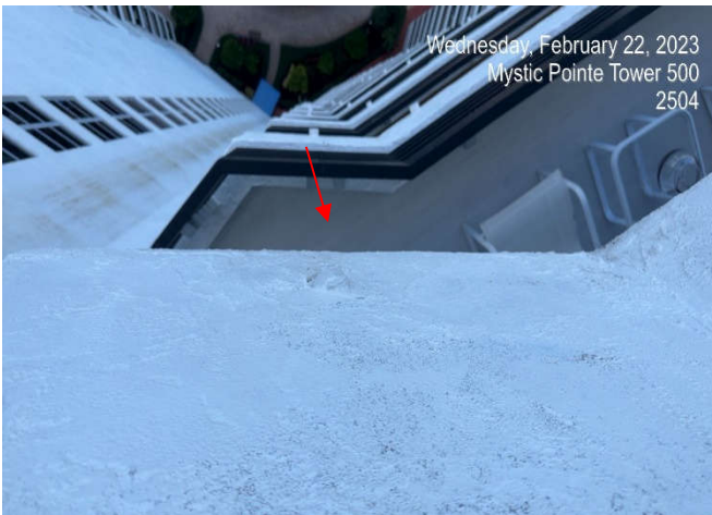
Photo 7.5.3 – Broken scupper at the balcony (Unit 2504)
