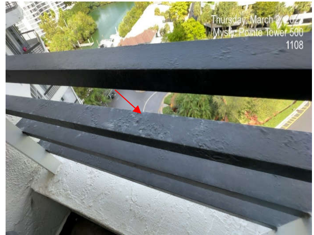
Photo 7.4.8 – Pitting and blisters at the balcony railing (Unit 2001)
