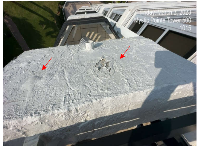
Photo 7.2.a.2 – Peeling and blistering paint at balcony knee wall (Unit 1015)
