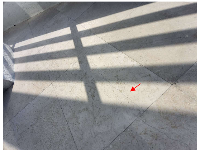
Photo 7.2.b.2 – Cracked tiled at balcony floor (Unit 2805)
