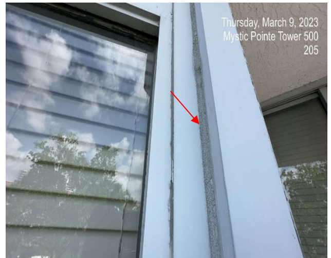
Photo 7.3.b.2 – Deteriorated metal-to-metal caulking at window (Unit 205)
