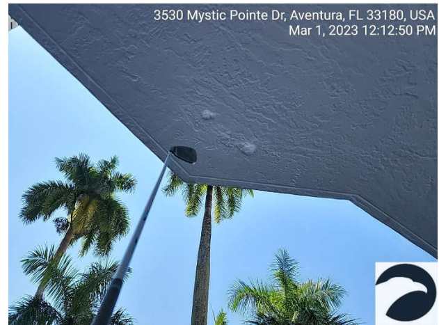
Photo 7.2.c.30 – Cracked stucco and initial stage of detachment at Pool Deck ceiling (Unit 903)
