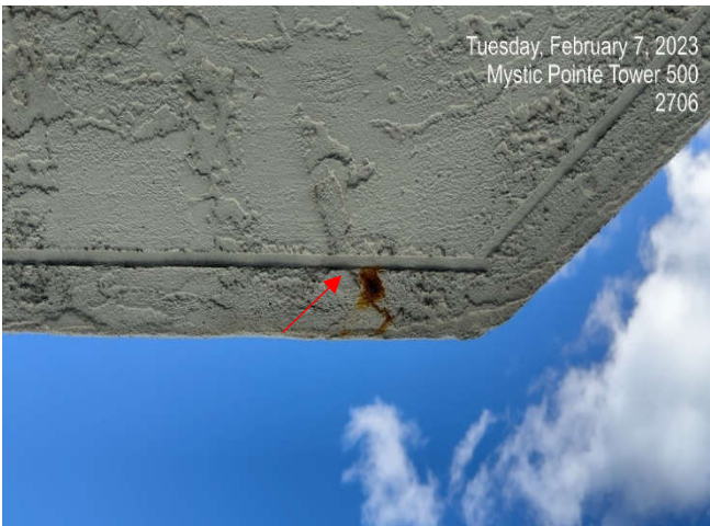
Photo 7.1.b.1 – Rust spot at the balcony ceiling (Unit 2706)
