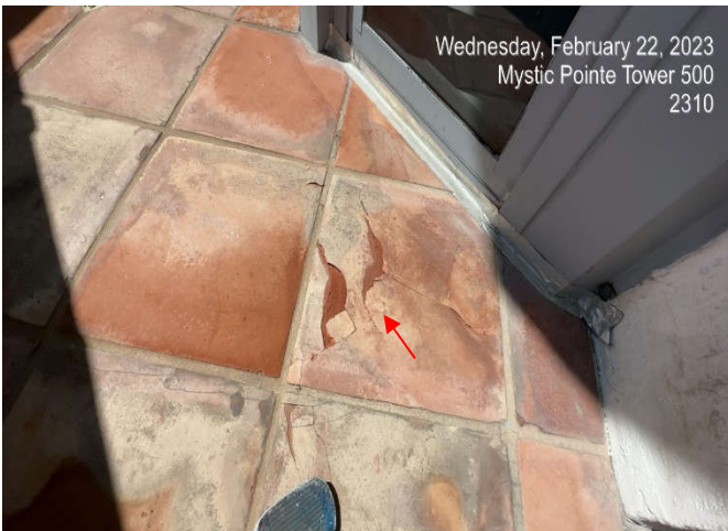
Photo 7.2.b.1 – Hollow and cracked tile at balcony floor (Unit 2310)
