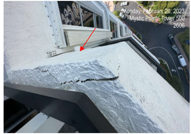
Photo 7.1.a.6 – Cracked concrete and hollow sound at balcony knee wall (Unit 2606)
