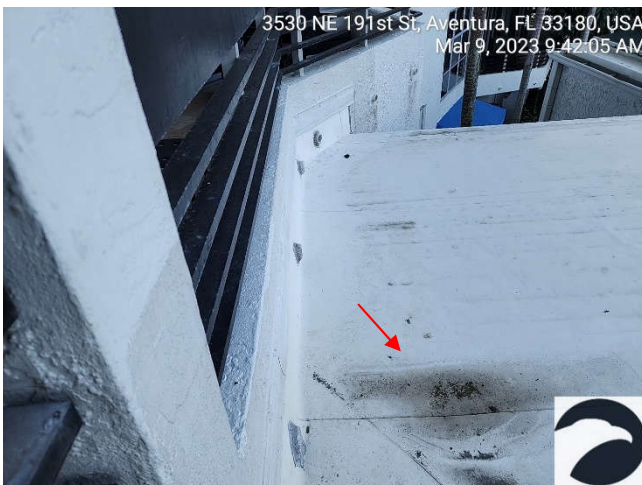
Photo 7.7.19 – Ponding water at the Lower Roof area
