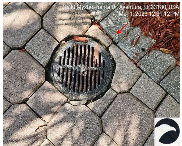
Photo 7.8.8 – Corroded drain cover at the Pool Deck
