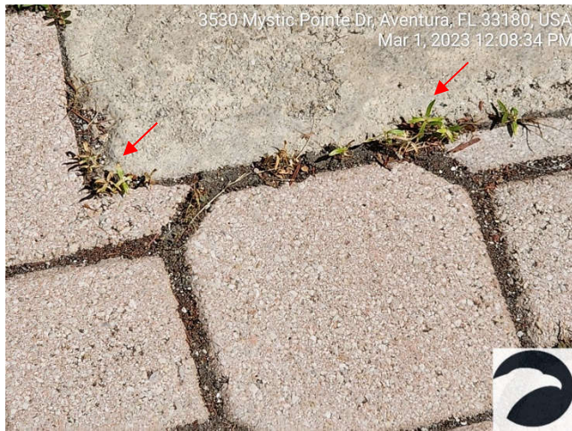
Photo 7.8.5 – Biological growth at paver joints (Pool Deck Level)
