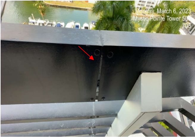
Photo 7.4.13 – Gap between railing connection (Unit 703)
