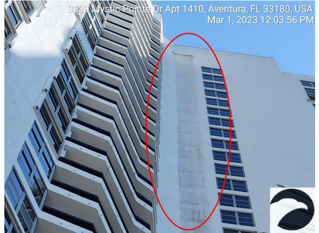
Photo 7.2.a.6 – Stained paint at exterior wall from the Mechanical Room Level (West Facade)
