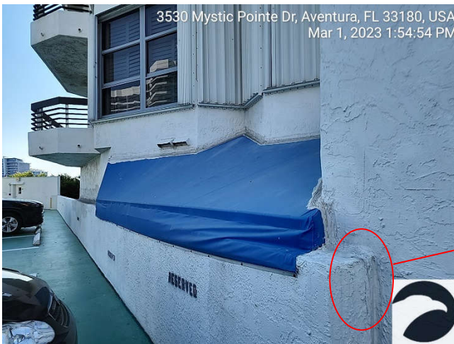
Photo 7.6.7 – Cracked expansion joint at the building façade (Garage Level 4)
