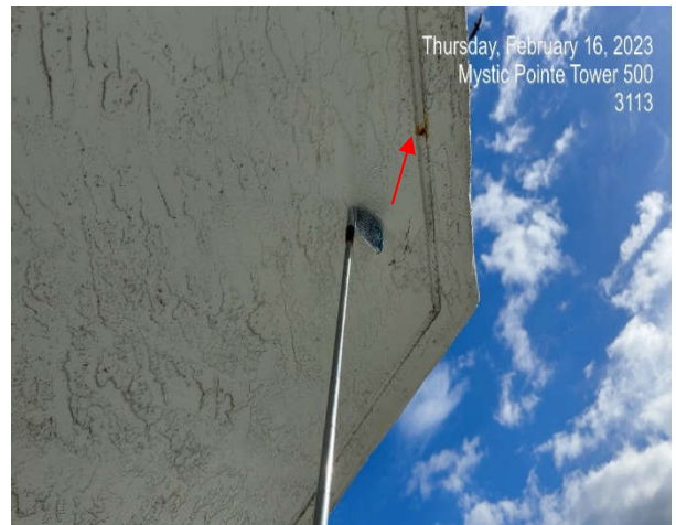
Photo 7.1.b.8 – Rust spot at the balcony ceiling (Unit 3113)
