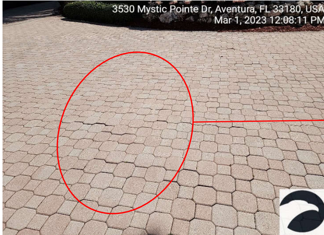
Photo 7.8.3 – Uneven pavers at the Pool Deck
