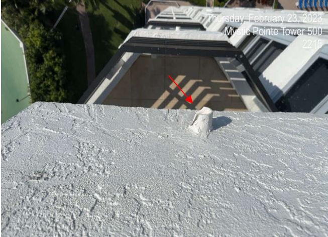
Photo 7.5.5 – Broken scupper (Unit 2215)
