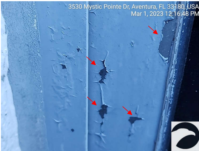
Photo 7.3.a.7 – Delaminated paint at Pool Deck storefront (Ground Level)
