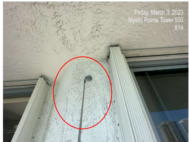
Photo 7.2.c.12 – Stucco delamination at balcony wall (Unit 814)
