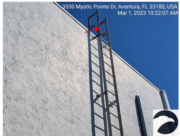
Photo 7.7.14 – Corroded ladder (Main Roof)
