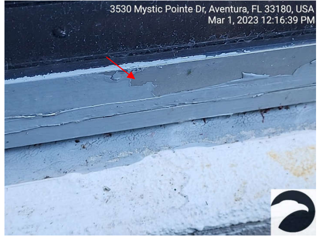
Photo 7.3.a.6 – Paint delamination at window frame (Unit 308)
