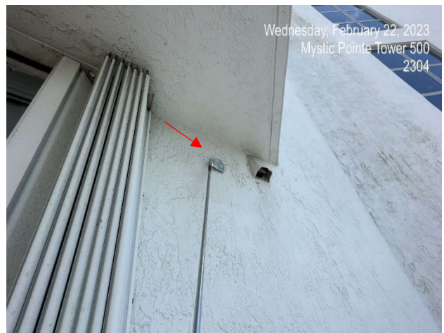
Photo 7.2.c.8 – Hollow sound and stucco delamination at balcony wall (Unit 2304)
