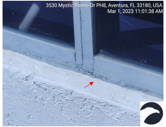
Photo 7.3.b.8 – Deteriorated metal-to-metal sealant at window (Unit PH-8)
