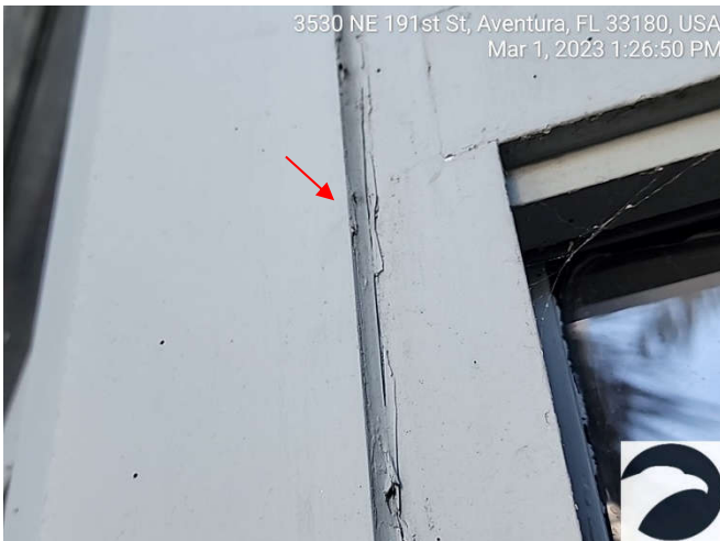
Photo 7.3.b.9 – Deteriorated metal-to-metal sealant at window (Unit 308)
