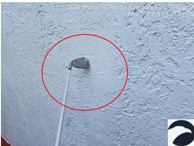
Photo 7.2.c.31 – Stucco delamination, hollow sound at building wall (Pool Deck Level)
