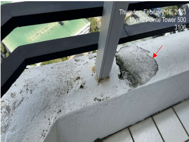
Photo 7.2.a.1 – Peeled paint and mold at balcony knee wall (Unit 3106)
