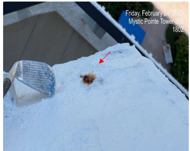
Photo 7.1.b.16 – Rust spot at balcony knee wall (Unit 1802)
