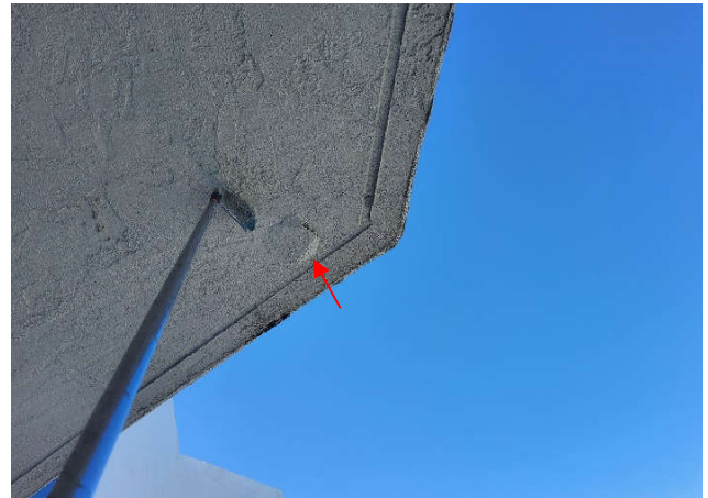
Photo 7.2.c.18 – Initial stage of stucco detachment at balcony wall (Unit 814)
