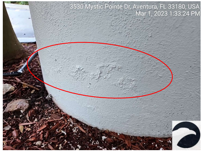
Photo 7.2.a.8 – Peeling and blistering paint at column of the Entry Lobby (Ground Level)
