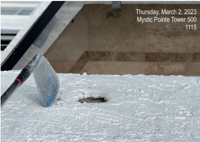
Photo 7.5.7 – Missing scupper (Unit 1115)
