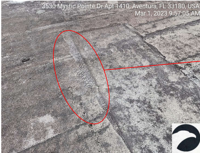
Photo 7.7.5 – Deteriorated and cracked roofing membrane at previous repair (Main Roof)
