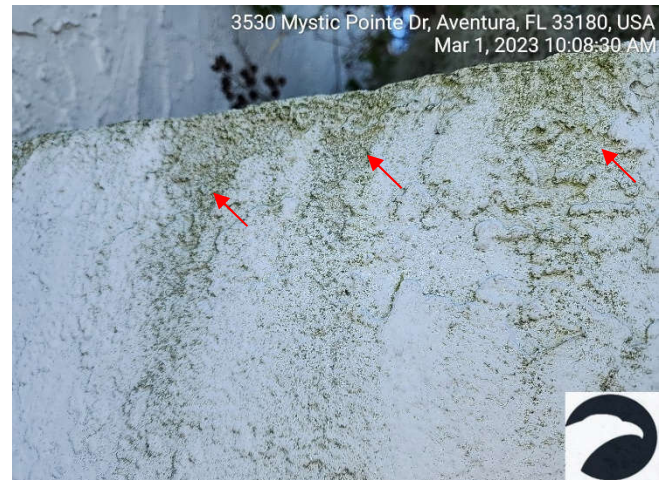
Photo 7.2.a.4 – Stained paint with biological growth at parapet wall (Roof Level)
