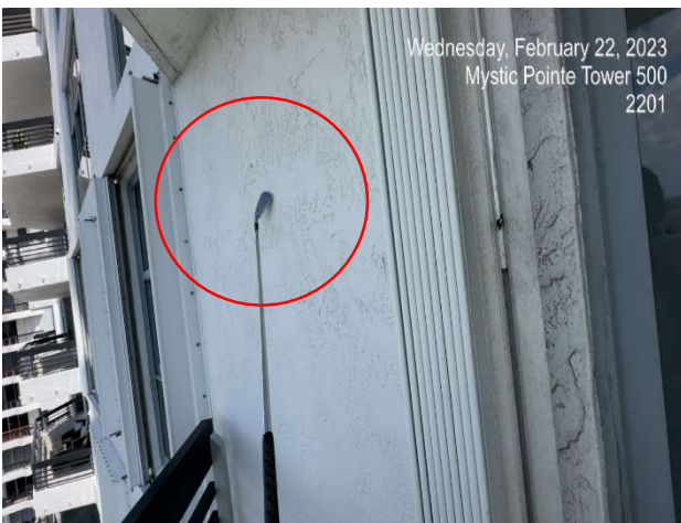
Photo 7.2.c.7 – Stucco with hollow sound at balcony wall (Unit 2201)
