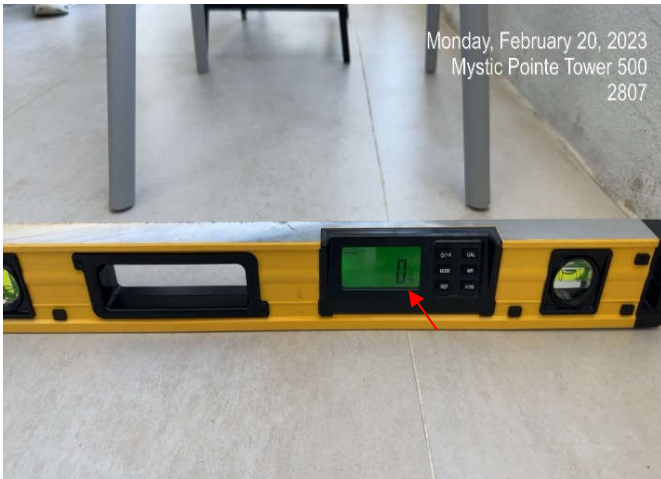
Photo 7.2.b.3 – Zero slope at the balcony floor (Unit 2807)
