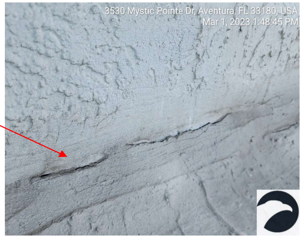
Photo 7.6.6 – Cracked expansion joint at the building façade (Garage Level 4)
