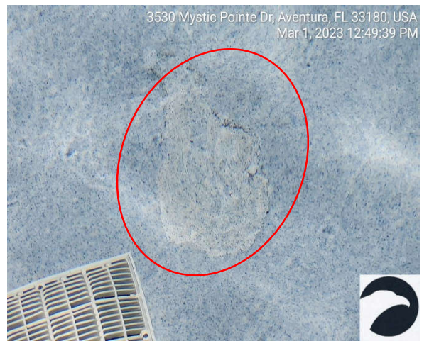
Photo 7.8.14 – Deteriorated finish surface at jacuzzi (Pool Deck Level)
