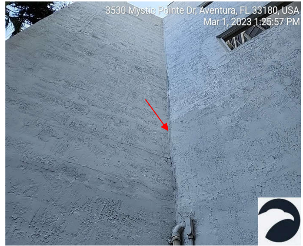
Photo 7.6.2 – Deteriorated expansion joint at the building facade (Lobby Level)
