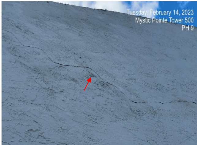
Photo 7.1.c.1–Stair-step crack at exterior CMU parapet wall (PH 09)
