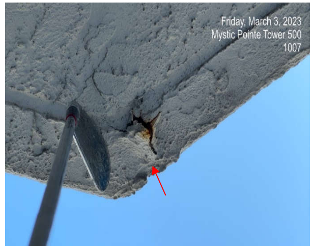
Photo 7.1.b.10 – Rust spot at balcony ceiling and initial stage of concrete / stucco delamination (Unit 1007)
