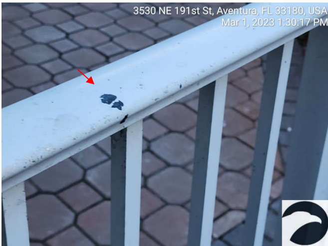
Photo 7.2.a.9 – Delaminated paint at Pool Deck railing (Ground Level)
