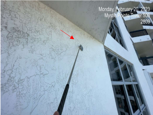
Photo 7.2.c.3 – Hollow sound and stucco delamination at balcony wall (Unit 2809)
