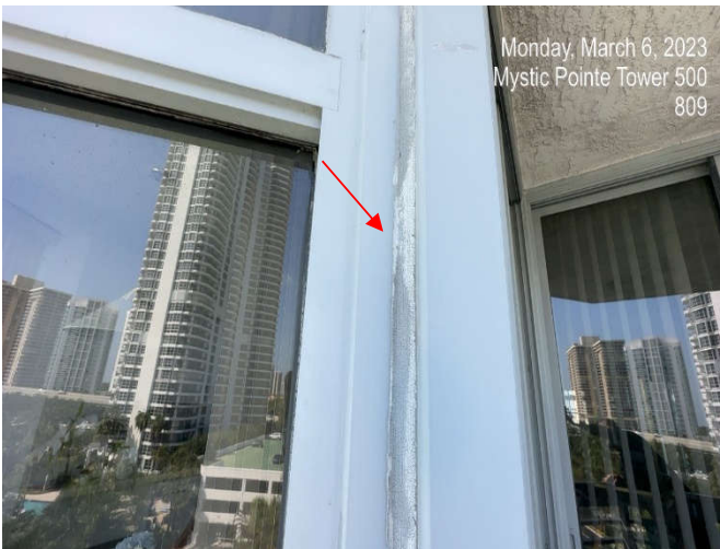
Photo 7.3.b.1 – Deteriorated metal-to-metal caulking at window (Unit 809)
