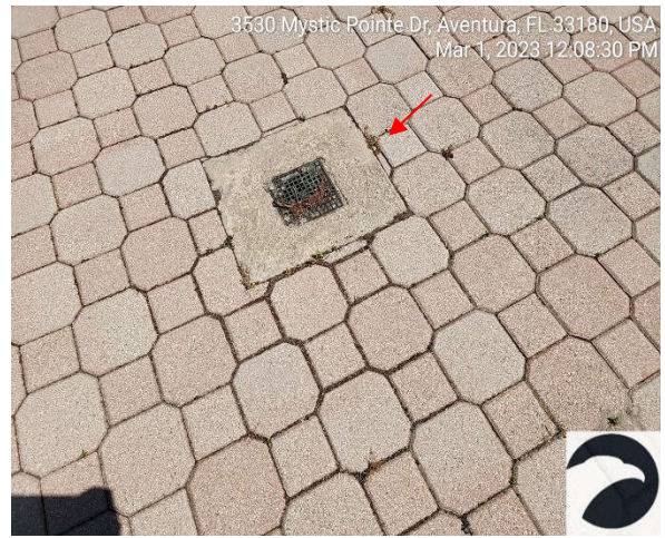
Photo 7.8.6 – Efflorescence at the Pool Deck
