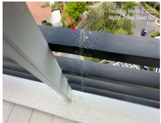
Photo 7.4.10 – Pitting and blisters at the balcony railing (Unit 1106)
