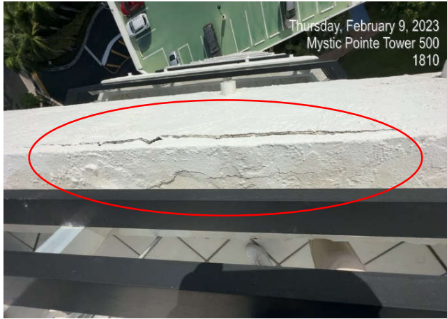
Photo 7.1. a.3 – Cracked concrete and hollow sound at balcony knee wall (Unit 1810)
