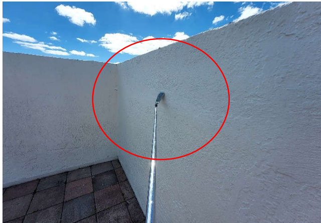
Photo 7.2.c.23 – Stucco delamination and hollow sound at parapet wall (Unit 1513)
