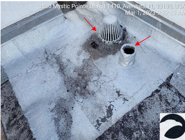
Photo 7.7.7 – Deteriorated previous repair performed around the drain (Main Roof)
