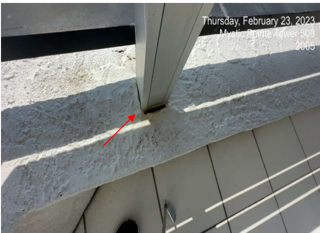
Photo 7.4.9 – Void around railing post (Unit 2005)
