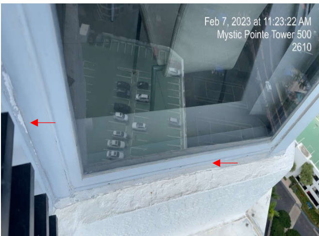
Photo 7.3.b.3 – Cracked and deteriorated stucco-to-metal and metal-to-metal caulking at window (Unit 2610)
