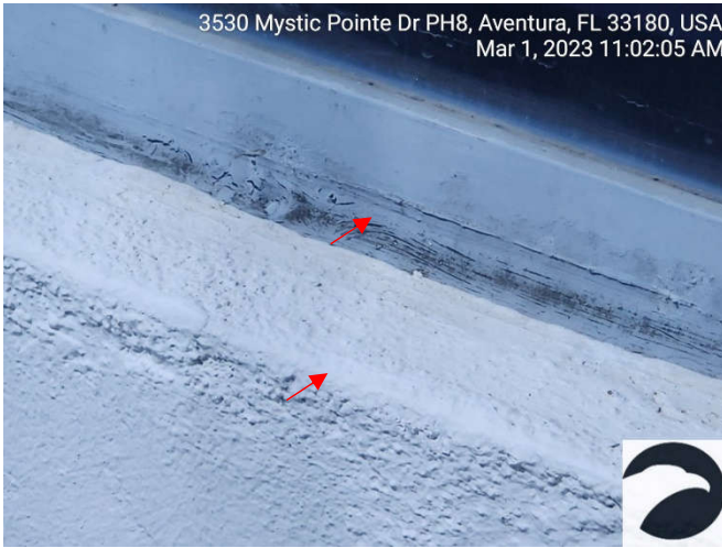
Photo 7.3.b.7 – Deteriorated metal-to-metal sealant at window (Unit 1407)
