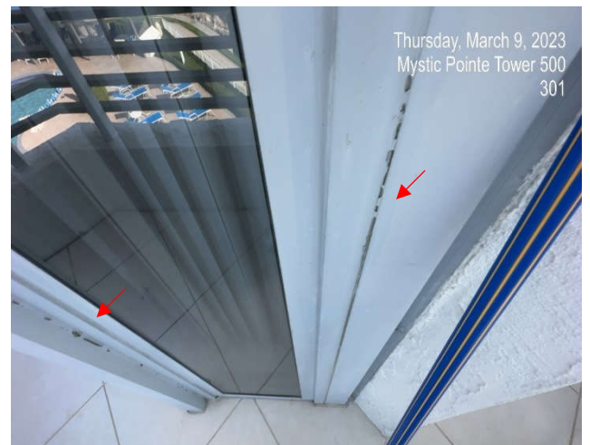
7.3.a.4 – Paint peeling at window (Unit 301)
