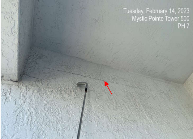
Photo 7.2.c.15 – Cracked stucco at balcony wall (PH 07)
