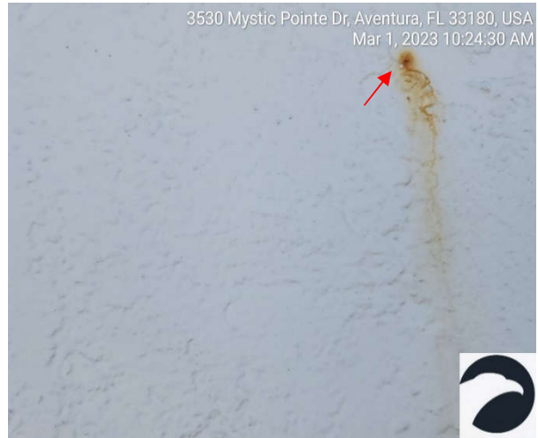
Photo 7.1.b.20 – Rust spot at parapet wall (Roof Level)
