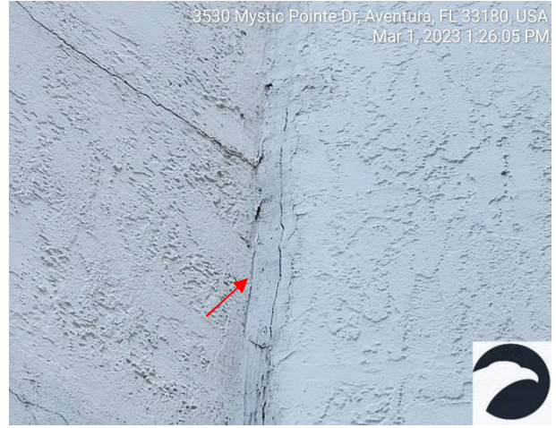
Photo 7.6.4 – Cracked expansion joint at the building façade (Lobby Level)
