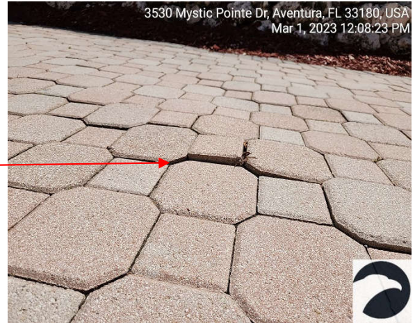
Photo 7.8.4 – Uneven pavers at the Pool Deck
