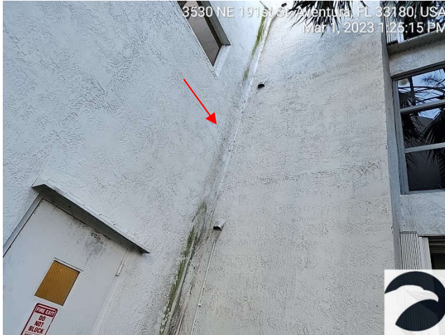
Photo 7.6.3 – Deteriorated expansion joint, with biological growth, at the building façade (Lobby Level)
