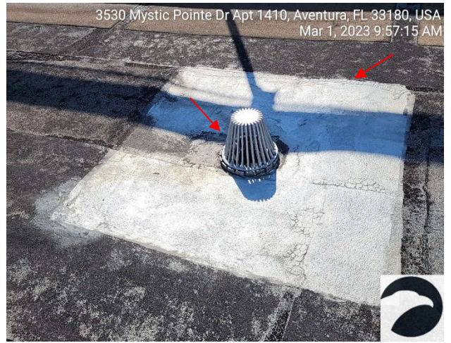
Photo 7.7.8 – Deteriorated previous repair performed around the drain (Main Roof)
