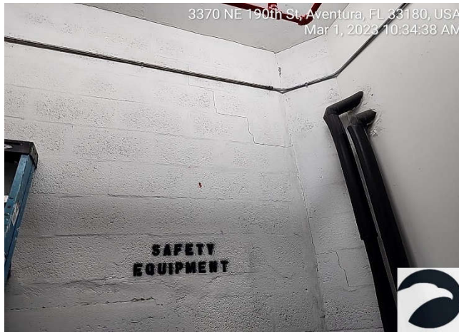
Photo 7.1.c.3 – Stair-step crack at interior CMU of the A/C Mechanical Room (Roof Level)
