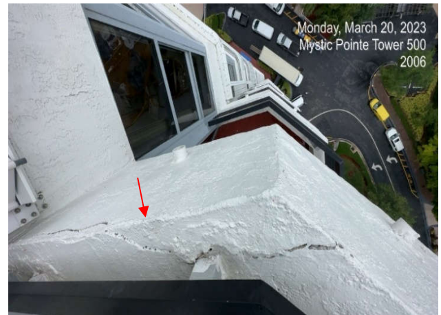
Photo 7.1.a.8 – Cracked concrete and hollow sound at balcony knee wall adjacent to the post pocket (Unit 2006)
