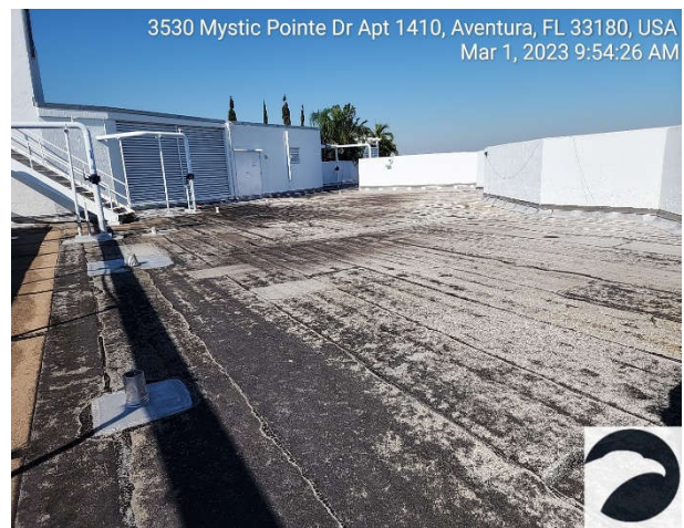
Photo 7.7.2 – Existing roofing system membrane in poor condition (Main Roof)
