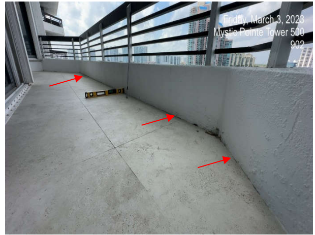
Photo 7.5.8 – Blocked scuppers (Unit 902)
