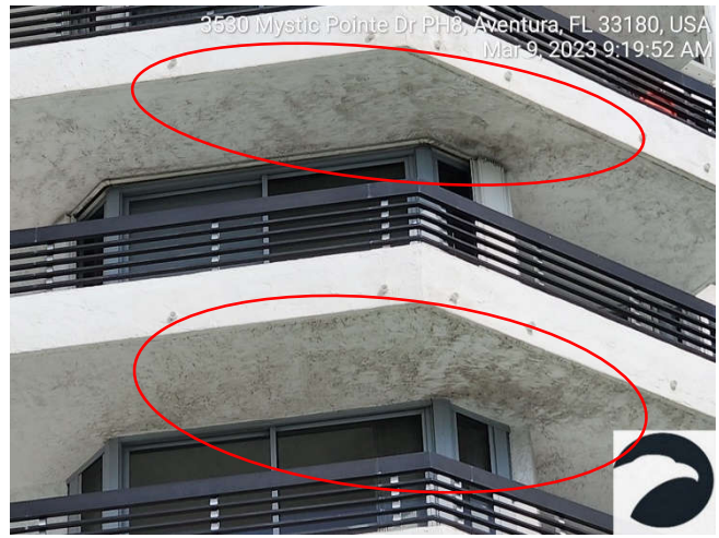
Photo 7.2.a.10 – Dirty paint at ceiling and walls of the balcony (West Facade)
