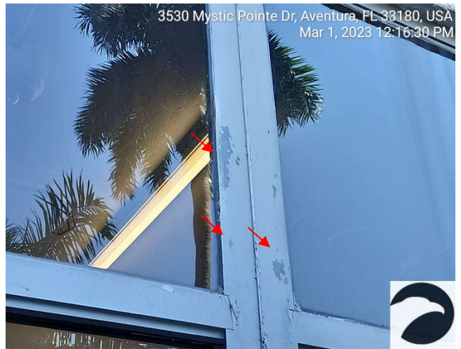
Photo 7.3.a.8 – Delaminated paint at Pool Deck storefront (Ground Level)
