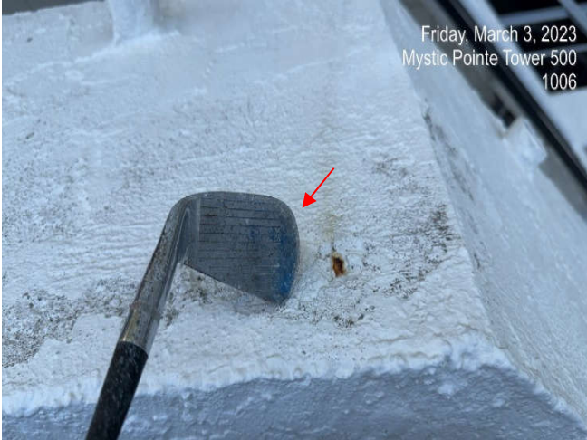
Photo 7.1.b.17 – Rust spot at balcony knee wall (Unit 1006)
