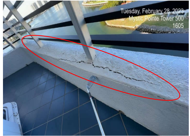
Photo 7.1.a.4 – Cracked concrete with hollow sound at balcony knee wall adjacent to the post pocket (Unit 1605)
