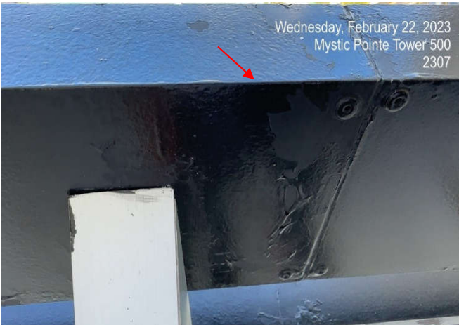
Photo 7.4.7 – Peeling paint at the balcony railing (Unit 2307)
