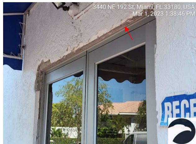
Photo 7.2.c.32 – Missing stucco at entrance door return (West Façade)
