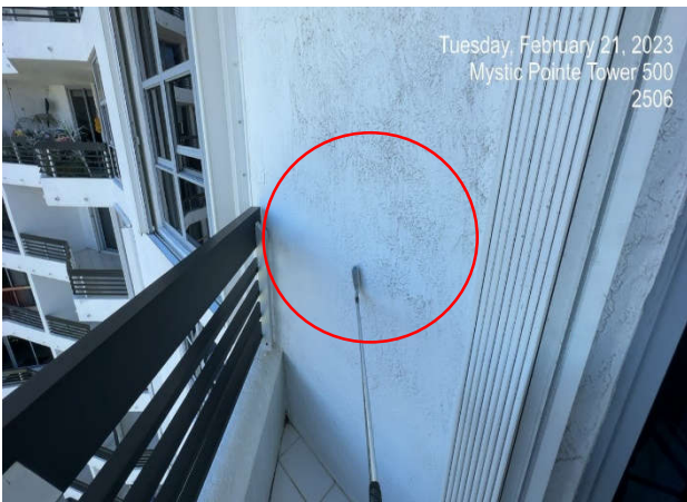
Photo 7.2.c.5 – Stucco with hollow sound at balcony wall (Unit 2506)
