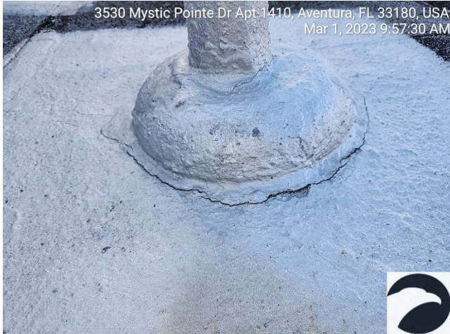
Photo 7.7.9 – Cracked and deteriorated sealant at the pitch pan and previous repair performed (Main Roof)
