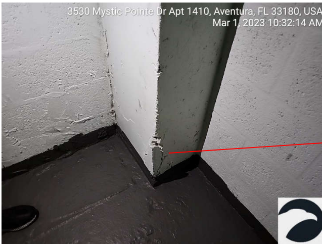
Photo 7.1.a.15 – Spalled concrete at column of the A/C Mechanical Room (Roof Level)
