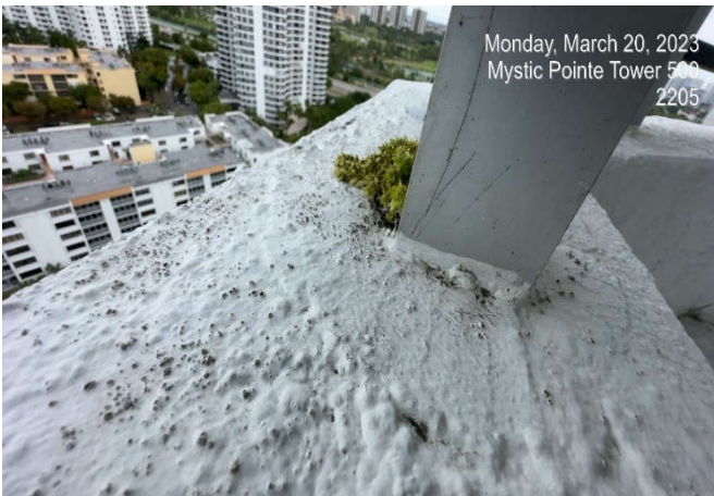
Photo 7.8.15 – Evidence of mold, biological growth at railing post pocket (Unit 2205)
