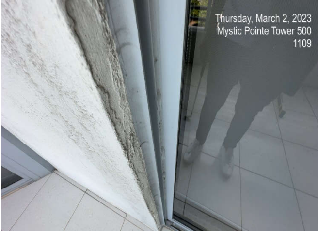
Photo 7.3.a.5 – Pitting at the sliding glass door frame (Unit 1109)
