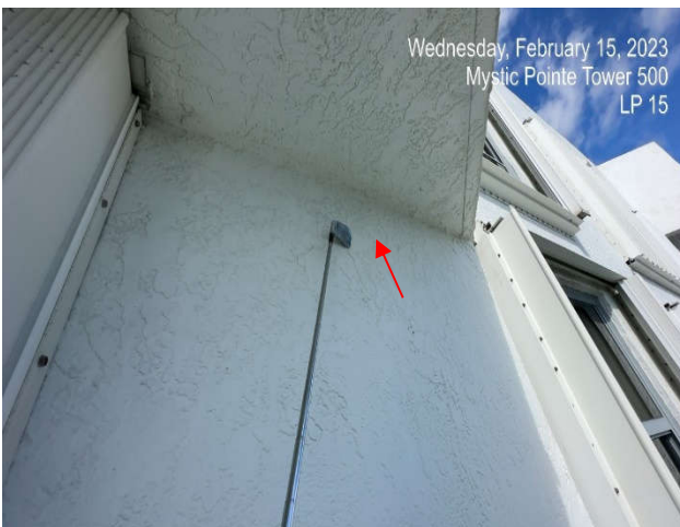
Photo 7.2.c.1 – Hollow sound and stucco delamination at balcony wall (LP 15)
