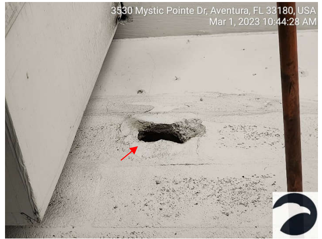
Photo 7.1.c.2 – Damaged CMU wall at interior of the A/C Mechanical Room (Roof Level)
