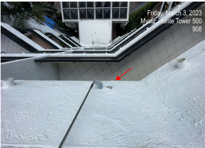
Photo 7.5.9 – Missing scupper (Unit 908)
