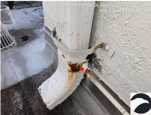
Photo 7.7.11 – Corroded downspout (Main Roof)
