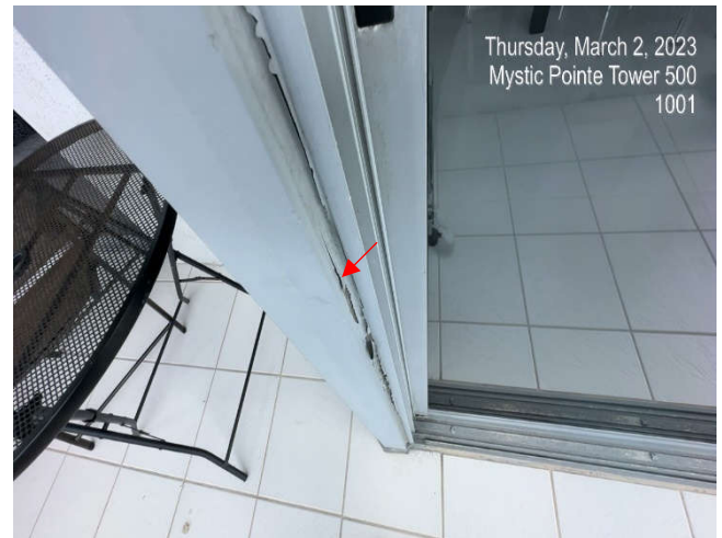
Photo 7.3.a.2 – Paint peeling at the sliding glass door (Unit 1001)
