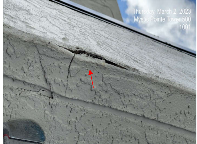
Photo 7.2.c.10 – Cracked and initial stage of detachment at ceiling of the balcony (Unit 1001)
