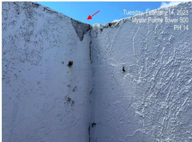
Photo 7.2.a.3 – Delaminated paint at CMU parapet wall (Unit PH 14)
