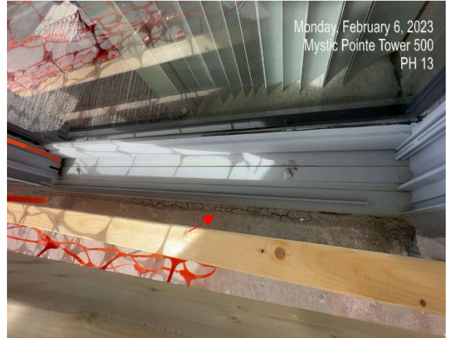
Photo 7.3.b.6 – Cracked and deteriorated stucco-to-metal caulking at the balcony sliding glass door sill (Unit PH 13)
