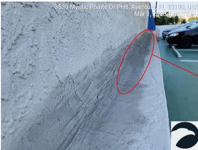
Photo 7.6.5 – Deteriorated and cracked expansion joint at the building façade (Garage Level 4)
