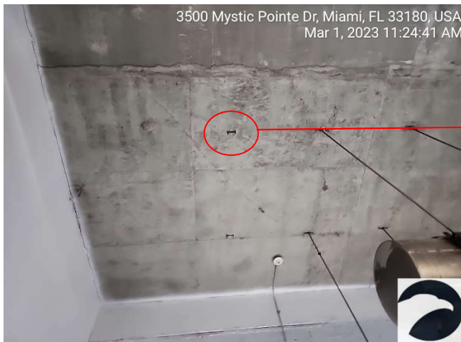
Photo 7.1.b.21 – Corroded embedded metal at ceiling of the Generator Room (Ground Level)
