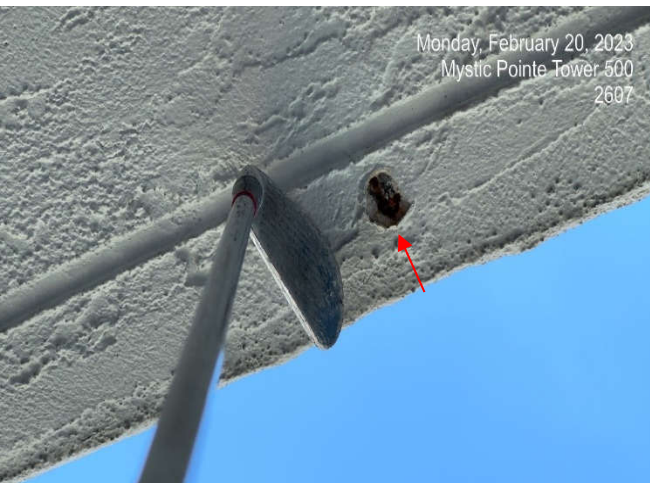
Photo 7.1.b.9 – Rust spot at the balcony ceiling (Unit 2607)
