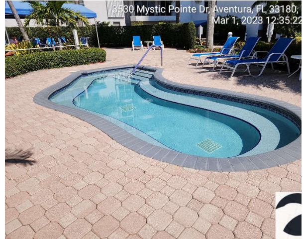
Photo 7.8.12 – Overall view of the jacuzzi in fair condition (Pool Deck Level)
