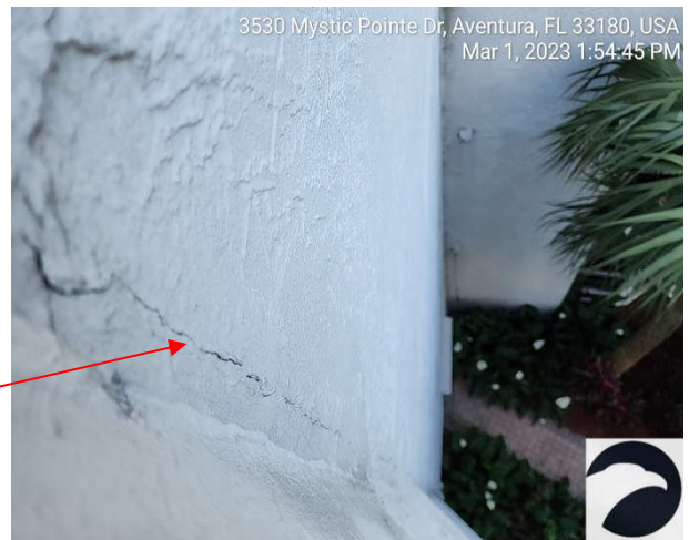
Photo 7.6.8 – Cracked expansion joint at the building façade (Level 4)
