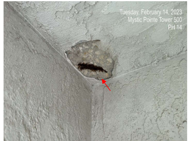
Photo 7.1.a.2 – Spalled concrete and exposed corroded rebar at the corner of balcony ceiling (PH 14)
