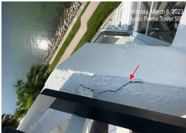
Photo 7.1.a.7 – Cracked concrete at balcony knee wall and hollow sound (Unit 815)
