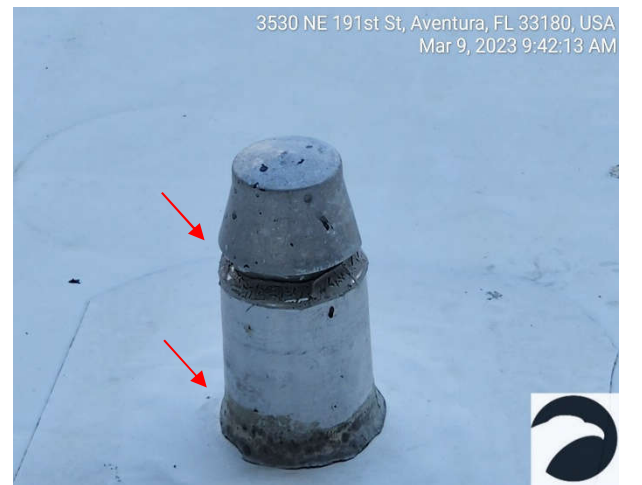
Photo 7.7.20 – Deteriorated and cracked sealant around the penetration of the roofing system (Lower Roof)
