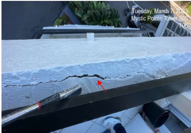
Photo 7.1.a.5 – Cracked concrete with hollow sound at balcony knee wall (Unit 706)
