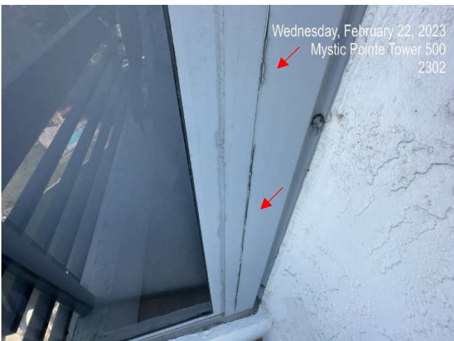
Photo 7.3.a.3 – Paint peeling at window (Unit 2302)
