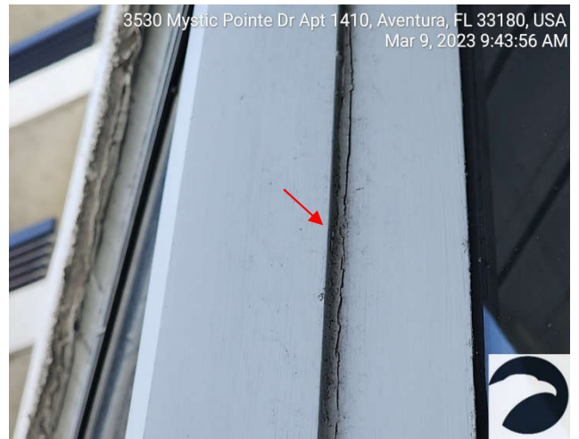
Photo 7.3.b.10 – Cracked metal-to-metal sealant at window (Unit 308)
