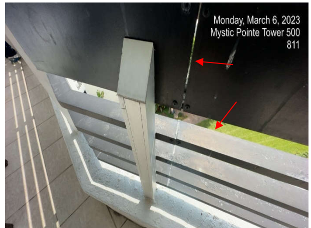
Photo 7.8.16 – Pitting, blisters, and gap between connection at the railing (Unit 811)
