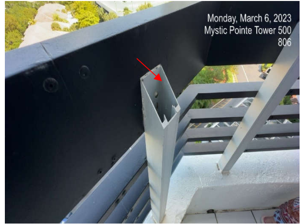
Photo 7.4.14 – Missing railing post cap (Unit 806)
