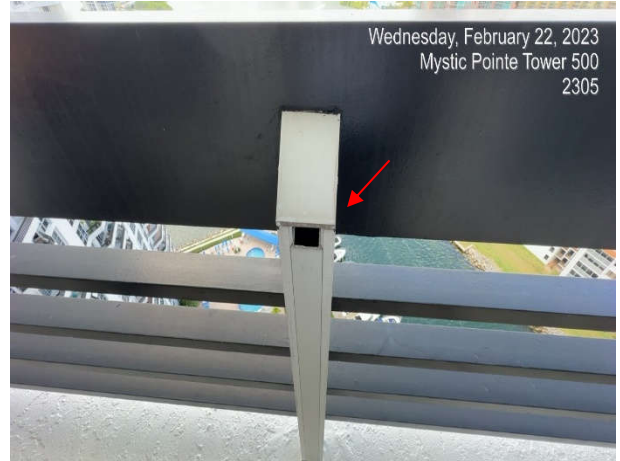
Photo 7.4.6 – Gap at the railing post (Unit 2305)
