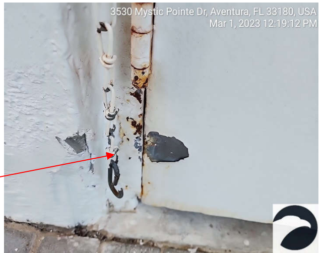
Photo 7.3.a.10 – Delaminated paint at Pool Deck storefront (Ground Level)
