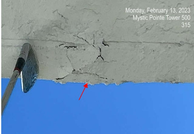
Monday, February 13, 2023 Mystic Pointe Tower 500 315 Photo 7.1.c.21 – Cracked stucco and initial stage of detachment at edge of the balcony ceiling (Unit 315)
