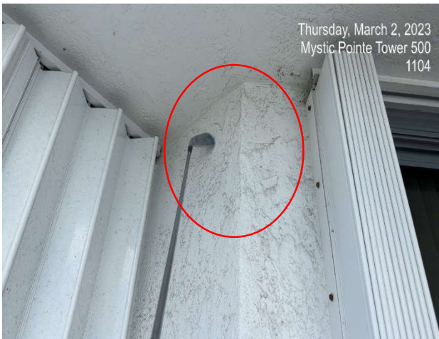
Photo 7.2.c.11 – Hollow sound and stucco delamination at balcony wall (Unit 1104)
