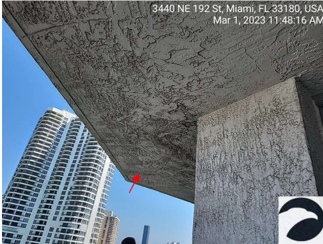
Photo 7.2.a.5 – Dirty paint at ceiling and walls of the balcony (Unit 3106)
