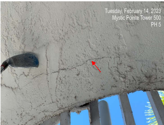
Photo 7.2.c.19 – Cracked stucco at balcony ceiling (PH 05)
