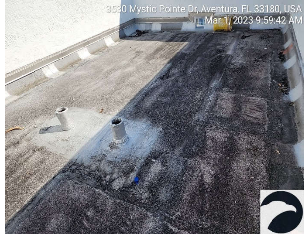
Photo 7.7.10 – Previous repair performed at multiple areas of the roof (Main Roof)
