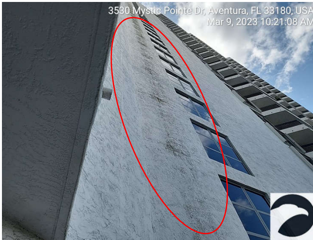
Photo 7.2.a.7 – Stained paint at exterior wall from the Mechanical Room Level (West Facade)
