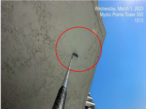
Photo 7.2.c.9 – Stucco with hollow sound at balcony ceiling (Unit 1513)
