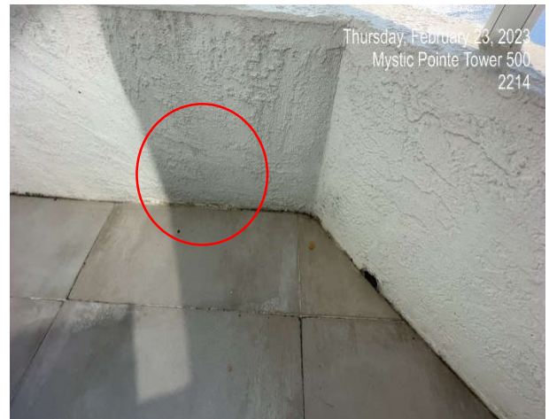
Photo 7.5.4 – Missing scupper hole (Unit 2214)
