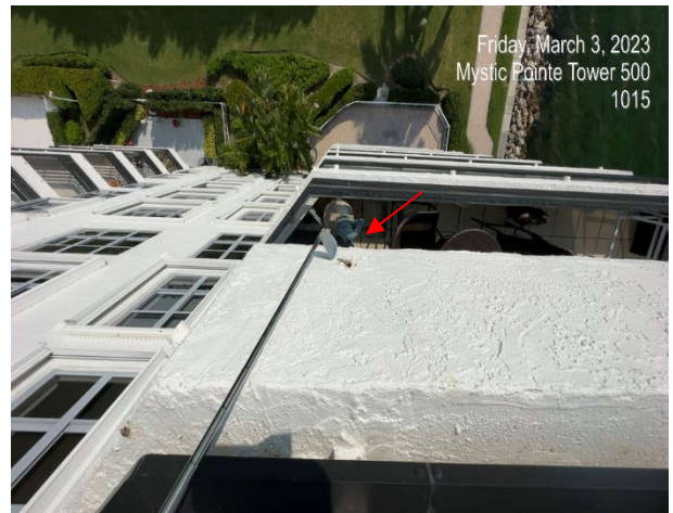
Photo 7.5.10 – Missing scupper (Unit 1015)
