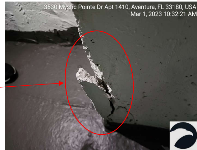
Photo 7.1.a.16 – Spalled concrete at column of the A/C Mechanical Room (Roof Level)
